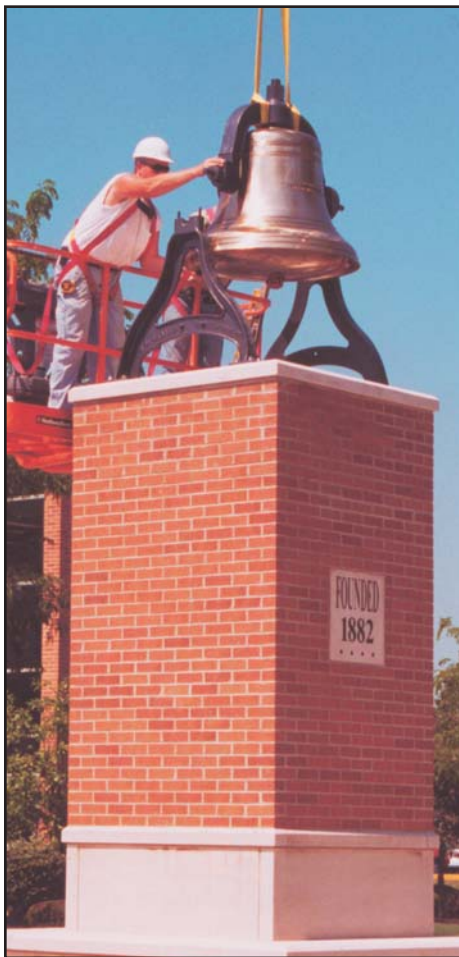
Construction workers mount the Old Main Bell on the newly built tower, located in the center of campus in front of the Gardner Fine Arts Pavilion.
