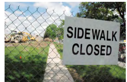
The sidewalk in front of the Davis Street Building is temporarily closed while construction crews work on the new building.
