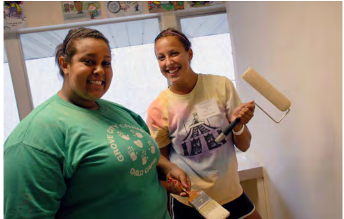
New students paint a classroom in the Findlay First Assembly of God on Ash Avenue.
